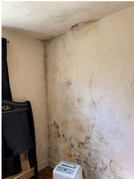
Mold covers a wall and ceiling at 85 Hawaii Avenue NE.
