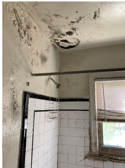
Mold growth on the ceiling and wall of a bathroom in 89 Hawaii Avenue NE.
