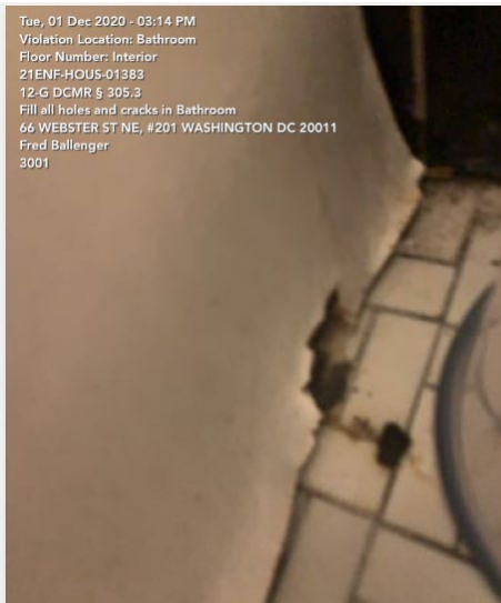
Holes in the wall at 66 Webster Street NE allow for ingress and egress of rodents.
