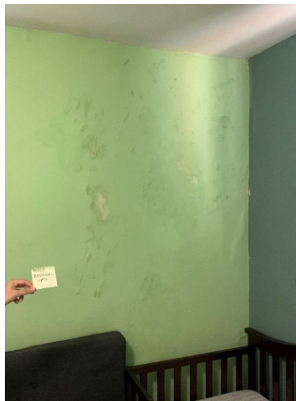
Mold covers the wall behind a crib at 73 Hawaii Avenue NE.
