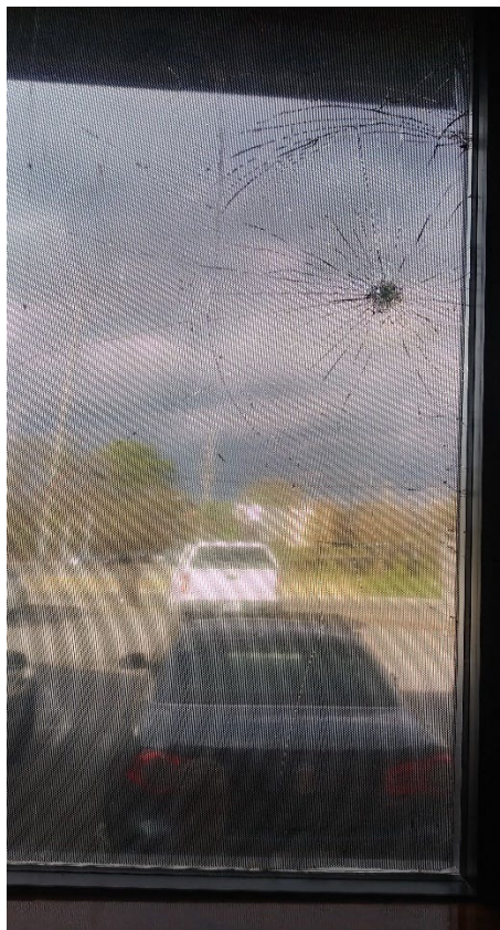
Shattered window at Creative Korner Early Learning Center, daycare in Alabama Plaza
